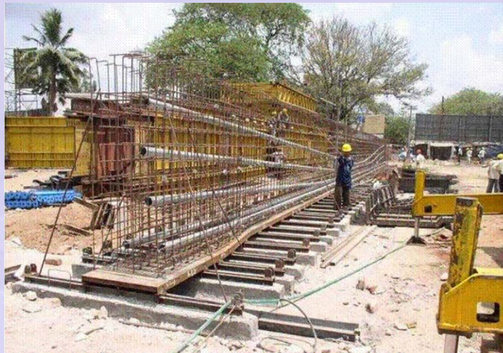
Figure 4-6.2 Tendon profiles in a simply supported bridge girder (Courtesy: Larsen & Toubro – Rambøll)
